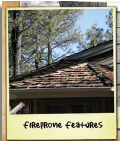
Use of flammable roofing materials
